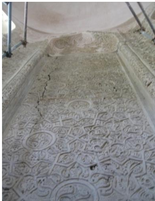
Fig. 7. Islimi designs and geometric patterns on the wall of the building, with visible structural cracks. (Photo by A. Moghaddasi)
