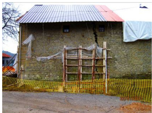
Damage to the North longitudinal wall
