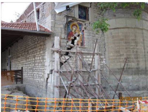
Damage to the South-East corner
