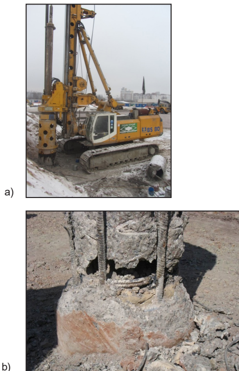
Figure 7. Pile construction with a casing pipe(a); a cavern in a drilled pile (b).
