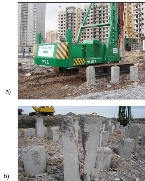
Figure 2. Pile driving equipment (a) and types of defects in driven piles (b).
