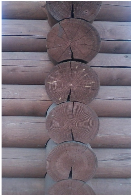
Figure 1. Crack on the surface of the technological notch
