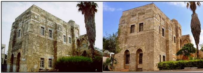
Figure 8. Northern building of the Pasha’s Palace complex before and after restoration (Ministry of Tourism and Antiquities, 2013).
