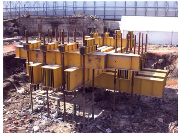
Fig. 1. General view of the loading platform for testing the piles with vertical static loading
