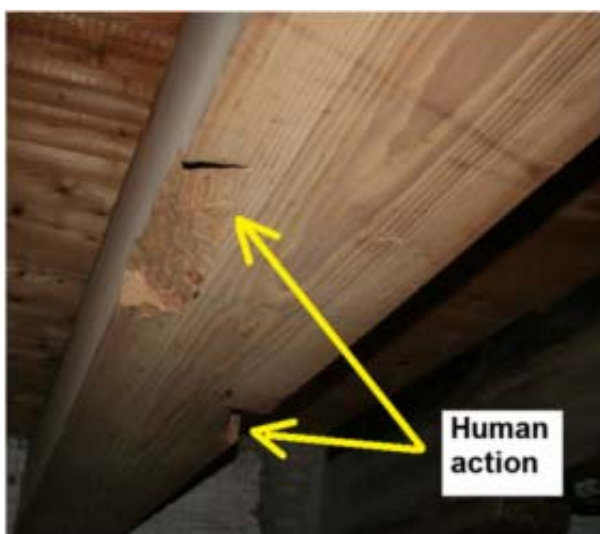
Fig. 2. Mechanical damage (Cabaleiro and Riveiro, 2016)
