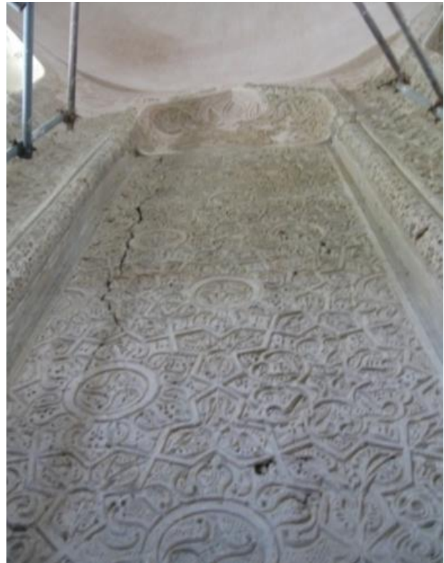
Fig. 7. Islimi designs and geometric patterns on the wall of the building, with visible structural cracks. (Photo by A. Moghaddasi)
