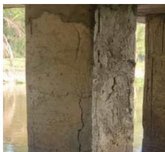
a) Cracks along the protective layer
