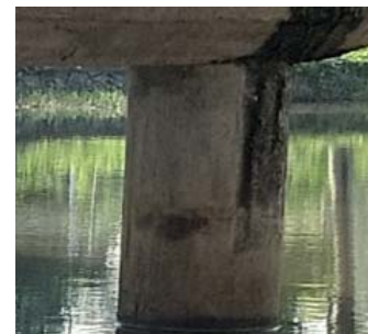
c) Rusty reinforcement revealed
