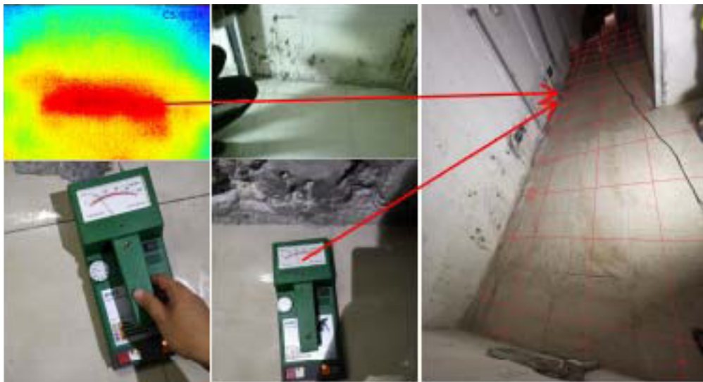
Fig. 9. Leakage point detection results for groundwater return in the wet-sticking decorative layer
