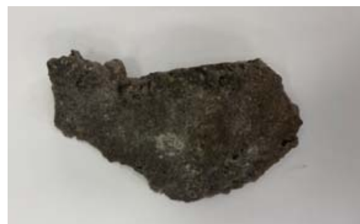
Fig. 8. Sample No. 2 of the plaster of the Main Treasury building in St. Petersburg
