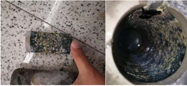
Fig. 20. Borehole coring at B10 after remediation for ground water return condition with regard to the wet-sticking decorative layer
