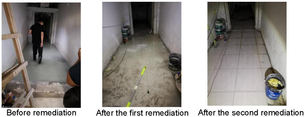
Fig. 18. Apparent effect after remediation for groundwater return condition with regard to the wet-sticking decorative layer
