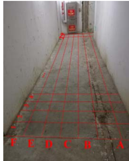
Fig. 6. Layout drawing of the groundwater return condition detection line without a decorative floor
