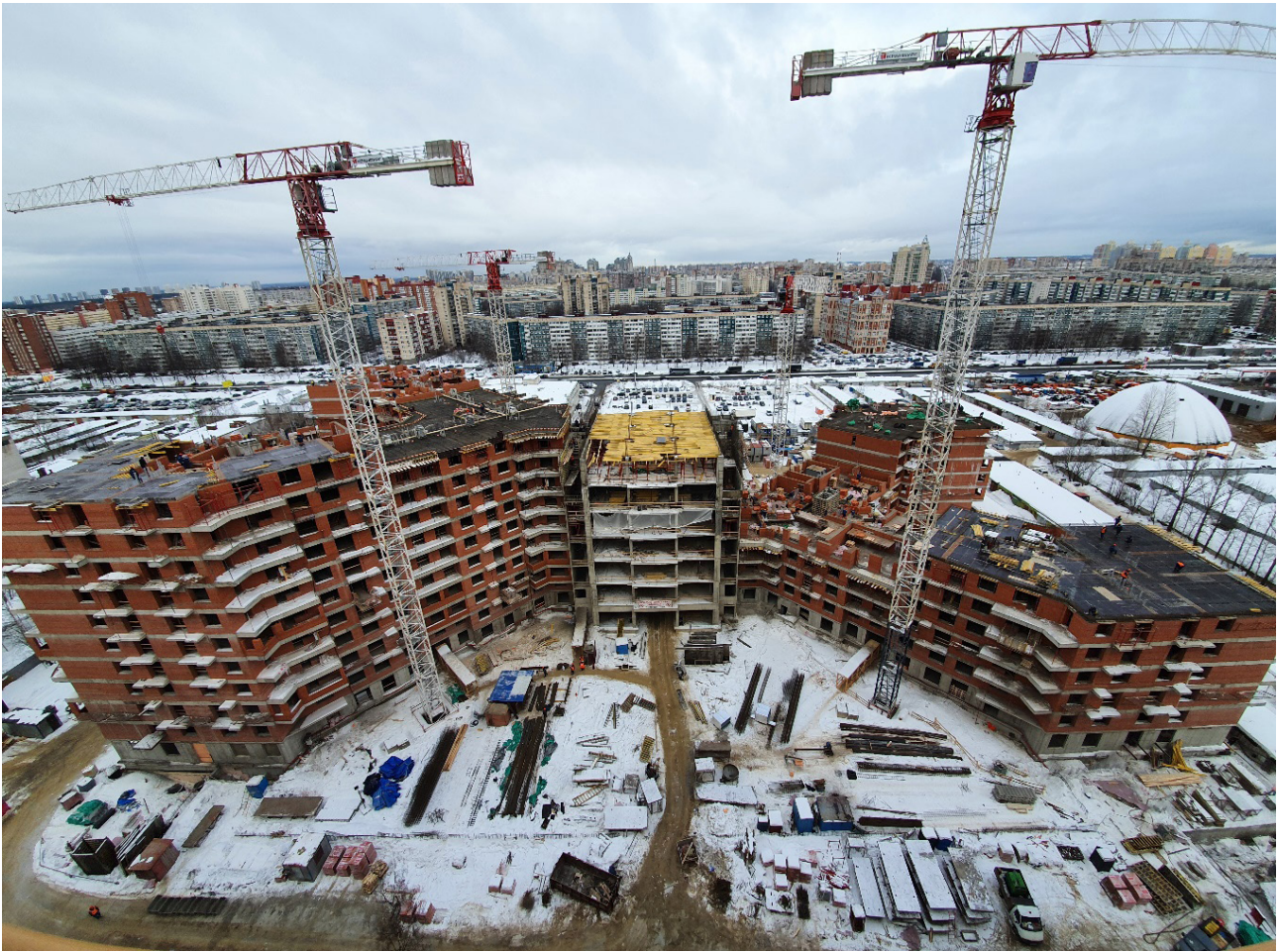
Figure 1. Construction of a multi-apartment residential building with integrated premises with the use of the cast-in-situ and precast technology. Saint Petersburg, 2022. Photo by O. A. Pastukh
