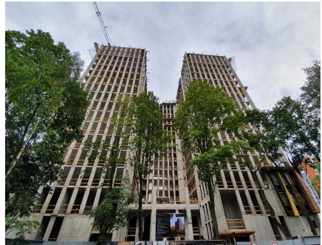
Figure 5. Construction of a multi-story residential building in Saint Petersburg (Legenda na Institutskom residential complex), 16 Institutsky Prospekt, (Legenda Intelligent Development, construction of the above-ground structures), 2020. Photo by A. N. Panin
