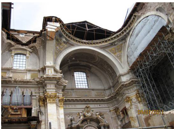
Figure 16. The church of St. Giorgio damaged by the 6 th of April 2009, L'Aquila-Italy, earthquake sequence (top and bottom)
