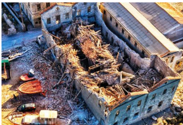
Figure 22. The partial collapse of one of the industrial buildings at the seafront of Karlovasi
