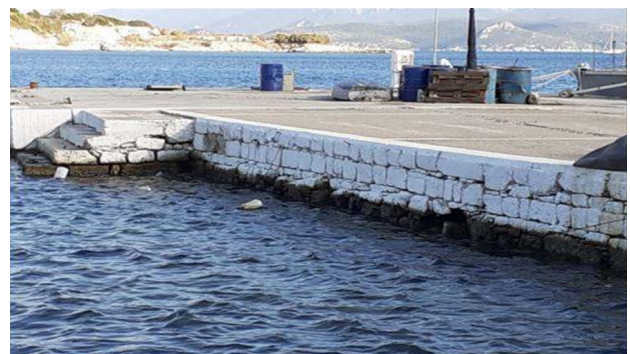
Figure 5. Permanent uplift of the embankment at the waterfront of Vathi
