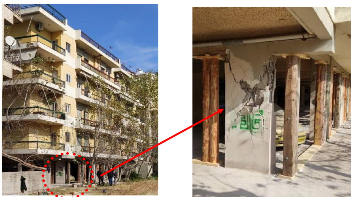
Figure 8. Shear failure of columns at the ground floor “soft” story of RC multi-story buildings at Samos island (ETAM report Nov. 2020 (Preliminary report, November 2020))
