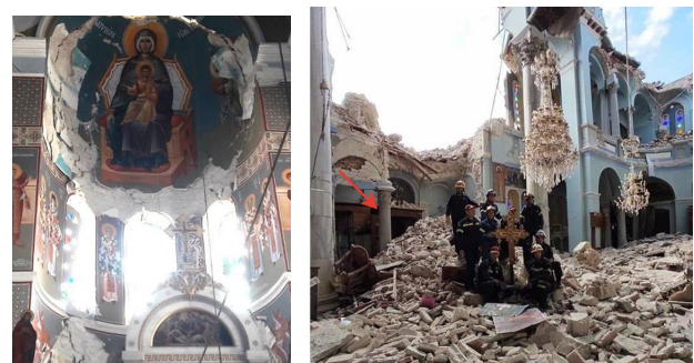
Figure 15. Damage of the Eastern peripheral wall with the Apse. Members of the emergency group salvaging the holy cross from the interior of this church
