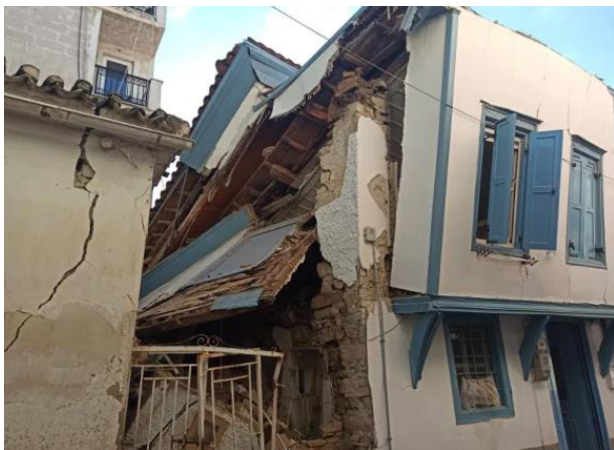
Figure 18. Damage of old low-story buildings at Vathi. In need of preservation because of particular architectural features
