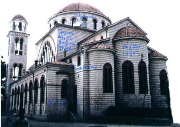
Figure 12. The church of St. Konstantinos and Eleni damaged by the 1999 Kozani-Greece earthquake (Manos et.al., 1997; Soulis and Manos, 2019)
