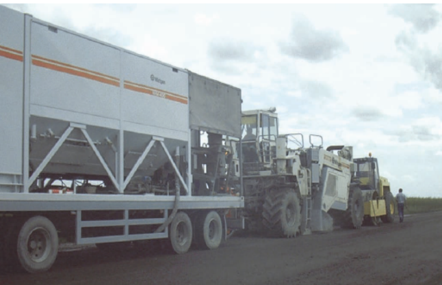
Figure 5. Construction of the base course with cold recycling (using WP-2500 recycler, with binder addition) (Federal Road Agency (Rosavtodor), 2016)
