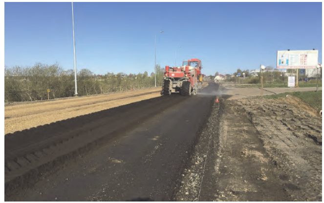
Figure 6. Cold recycling using WR-2500 Wirtgen recycler machines (complex binder: bitumen emulsion, cement) (Federal Road Agency (Rosavtodor), 2016)
