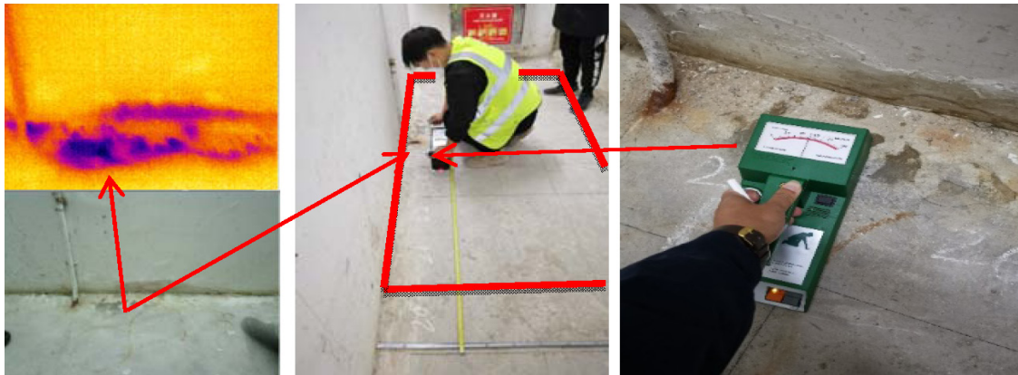
Fig. 7. Results for the groundwater return condition detection line without a decorative floor for leakage point detection
