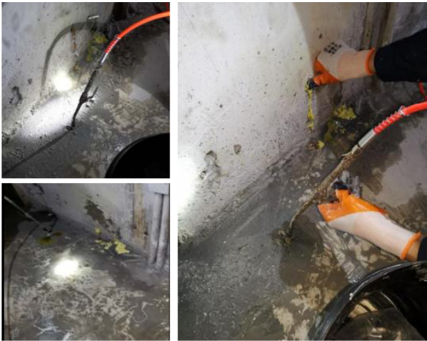
Fig. 17. On-site grouting remediation for groundwater return condition with regard to the wet-sticking decorative layer
