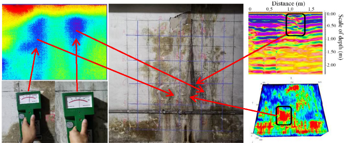
Fig. 12. Results of combined detection of side wall leakage without a decorative layer
