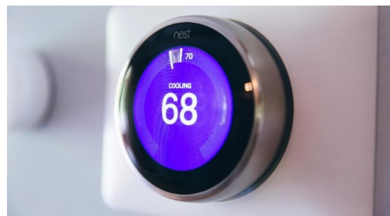
Fig. 1. AI Nest Thermostat device keeping the building at an optimal temperature (Wollerton, 2018)
