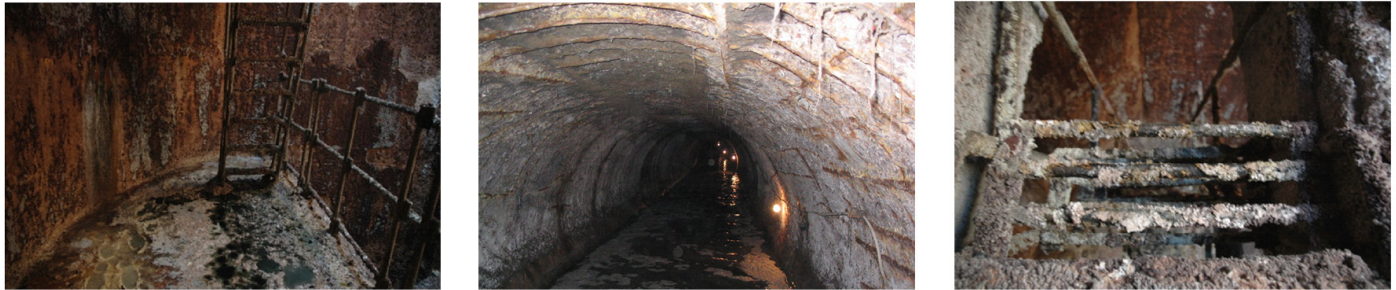
Figure 1. Corroded sewer shafts and collectors in St. Petersburg
