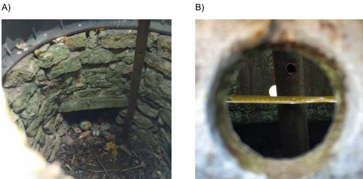
Figure 4. Examination of the inner cavity of the fountain: A) service opening, B) vertical pipeline
