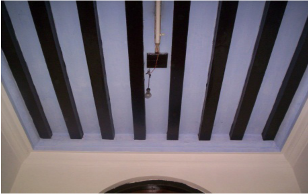
Figure 10. Heavy timber roof of traditional houses (Source: the author of the paper)
