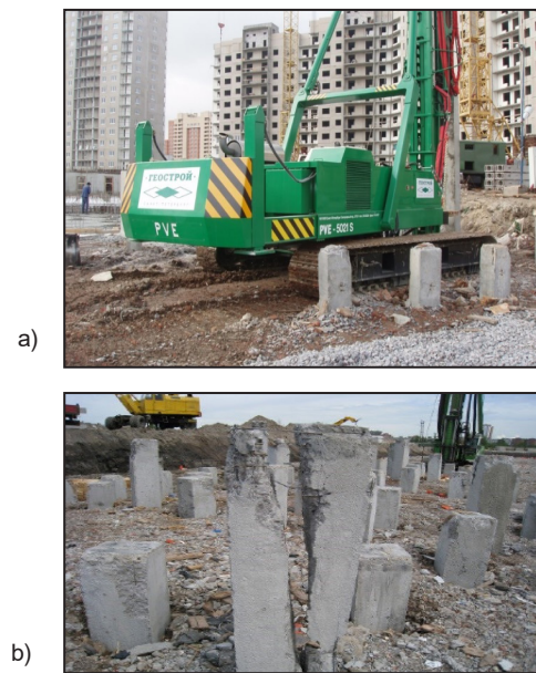
Figure 2. Pile driving equipment (a) and types of defects in driven piles (b).
