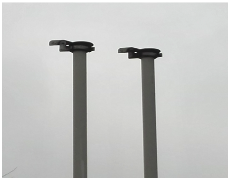
Figure 2. Standard termination of discharge and blowdown pipes at a Polish gas distribution unit plant
