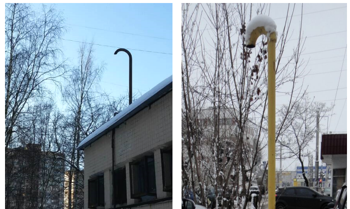
Figure 3. Standard termination of discharge pipes at Russian low-pressure GDPs.
