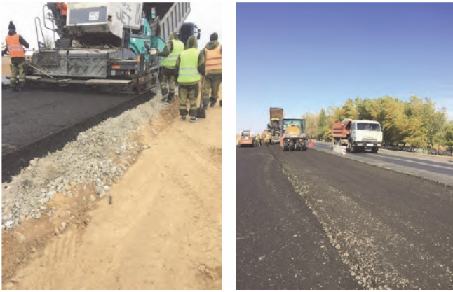
Figure 4. Construction of the base course with in-plant cold recycling (Federal Road Agency (Rosavtodor), 2016)
